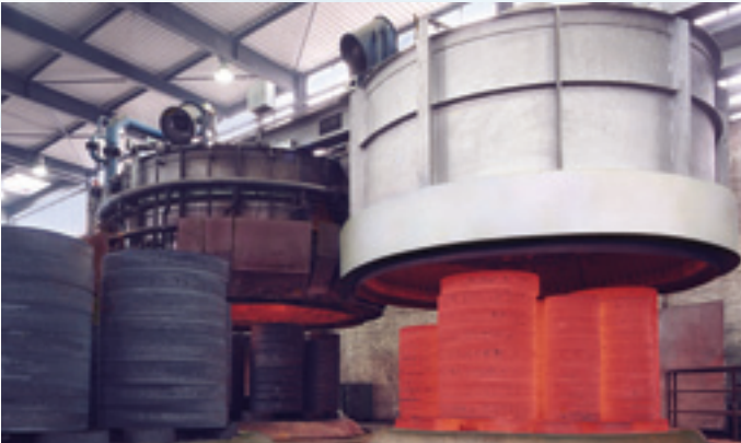
Bell-type annealing plant with 3 workstations
